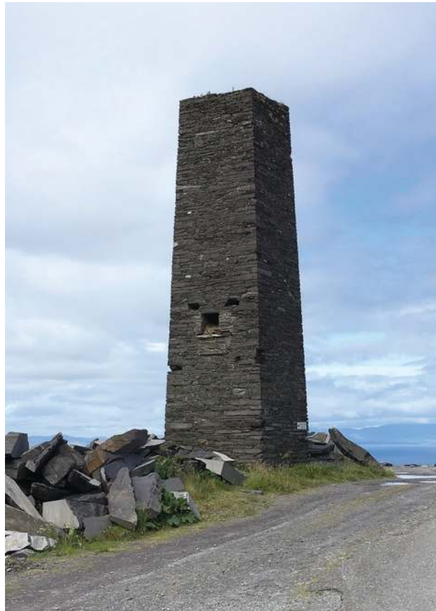
Fig. 6—Chimney at quarry site. It was attached to the squaring house to its immediate north; this was demolished in 1939.
